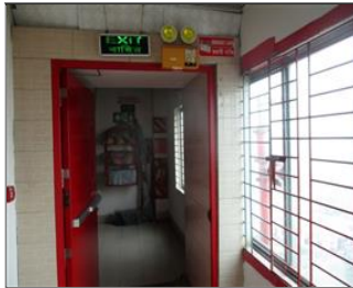
Photo of fire safety equipment Fire safety to confirm the sustenance-Fire rated door Exit sign Fog light.JPG
