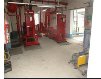
Photo of fire safety equipment Fire safety to confirm the sustenance-Fire hydrant pump.JPG
